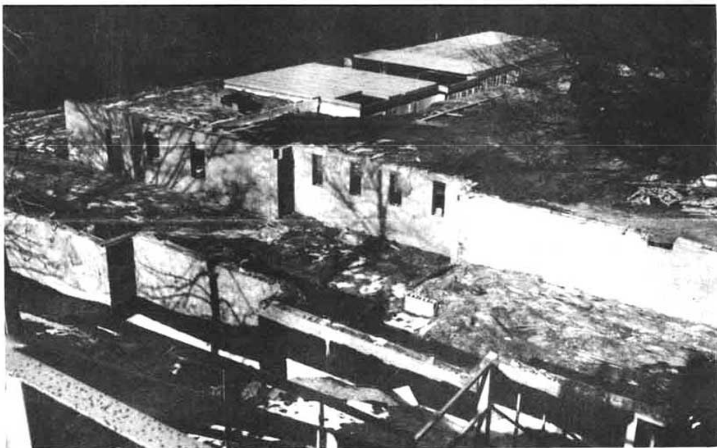
The view of the entire construction project from the main building of the seminary. In the foreground is the foundation for the new dormitory; in the distance is the construction work accomplished on the new chapel.
