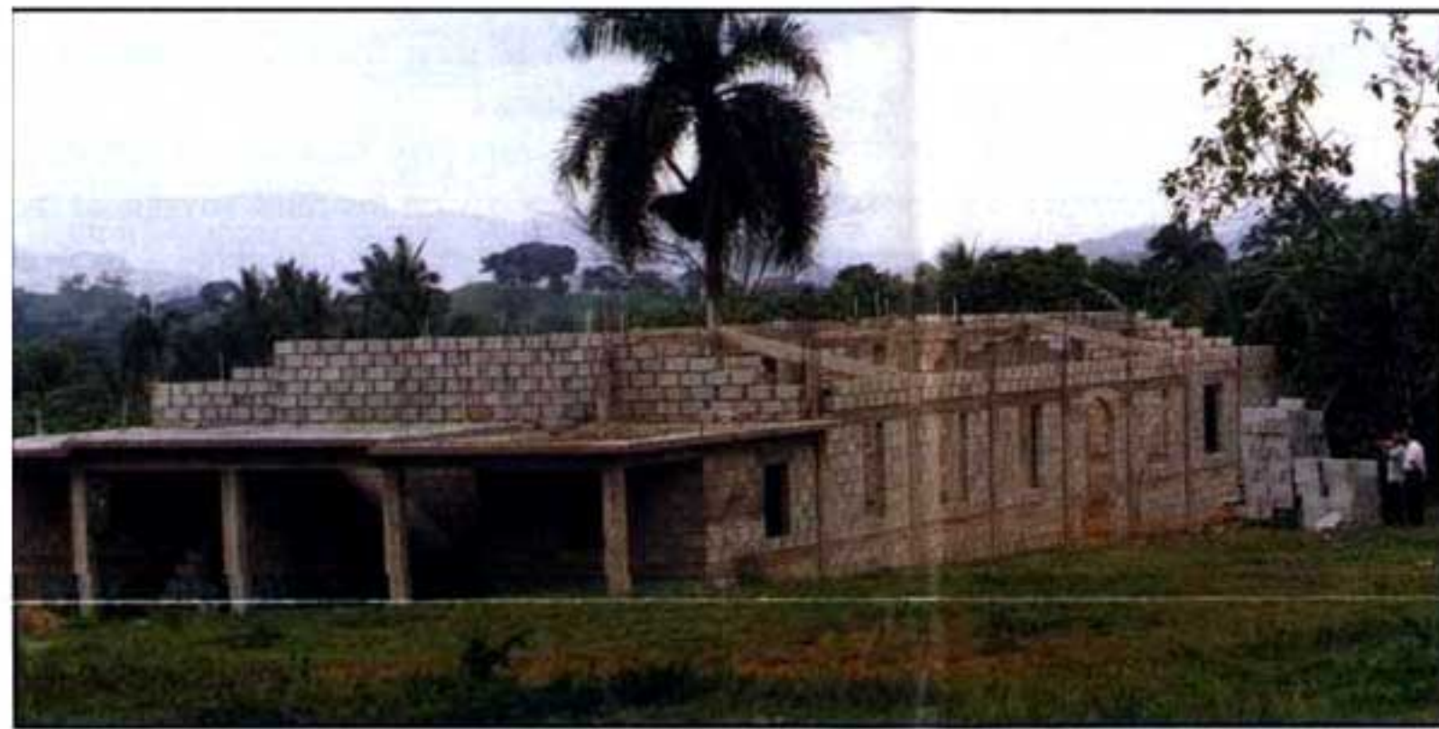
REBUILDING THE FAITH —In the countryside village of Yamasa (near Santo Domingo, Dominican Republic), a parish of 500 Traditionalist Catholics are building a church for the celebration of the true Mass, continuing the legacy of Columbus.
